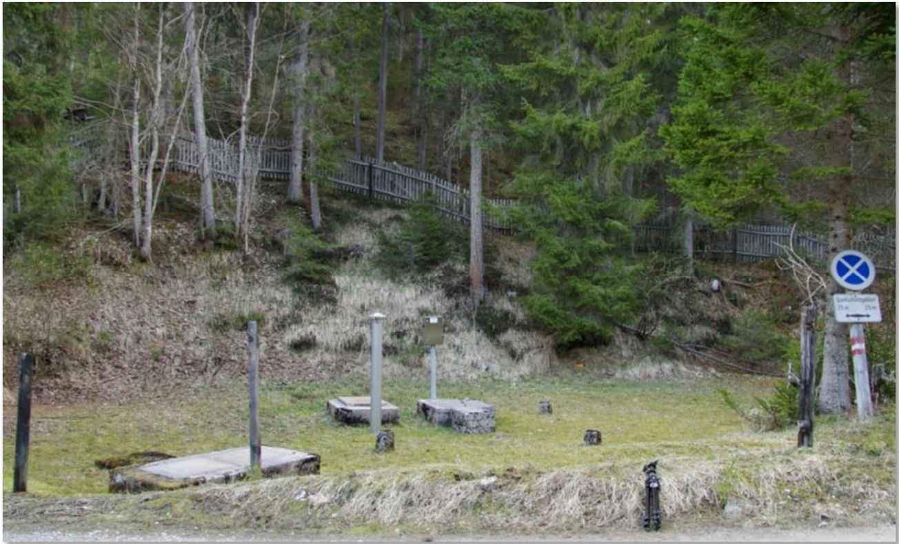
Fig 2: Initial situation of the Sagtümpel - the dilapidated drinking water complex. Photo: R. Seebacher
